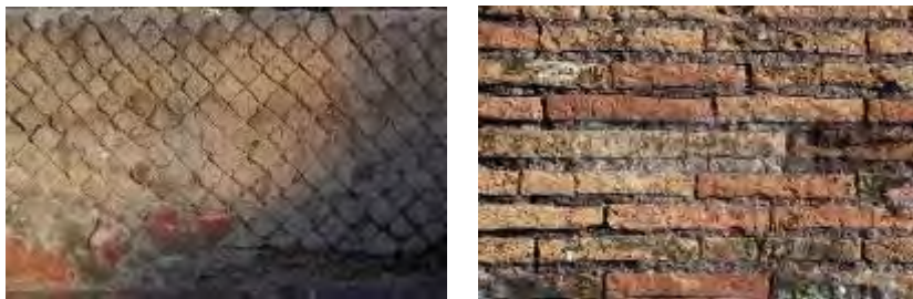
Figure 1.2: Stone masonry (Roman ruins of Abellinum, on the left) and brick masonry (Forum of Rome, on the right).
