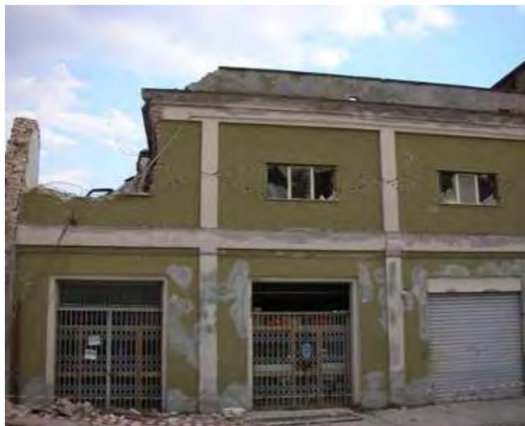
Figure 1.6: Partial collapse in a masonry building after L'Aquila earthquake [3].
