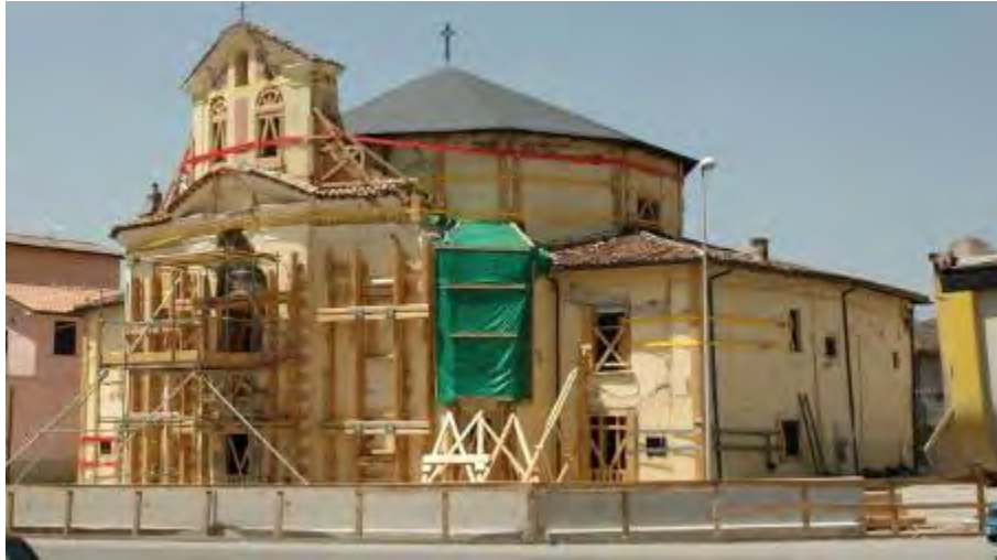
Figure 1.7: Interventions on a Church in L'Aquila to prevent other damages [3].
